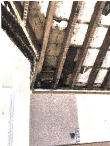
Cut back and treat decayed timber rafters in accordance with timber specialists report. Install treated new sister rafter and splice to existing with M10 staggered coach bolts with shear connectors.
