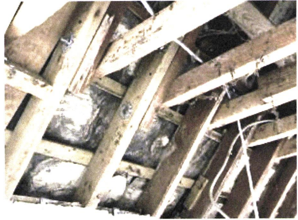
Remediate previous splicing which was found to be sub-standard. Install new sister rafters and splice with M10 coach bolts with shear connectors.
