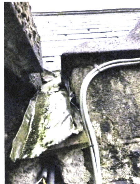
Replace defective and non-conforming gutter detail.
